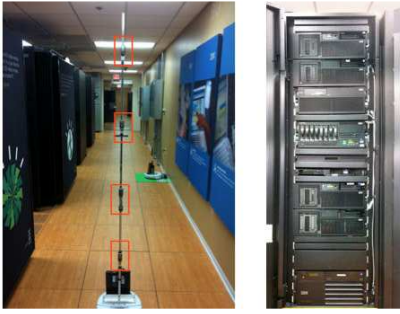
Figure 1: Our robot equipped with four forward-pointing cameras in addition to its downward-pointing camera, used for navigation, on the left, and the results of stitching images from the four cameras, on the right. The view is of a rack with rack door removed.
